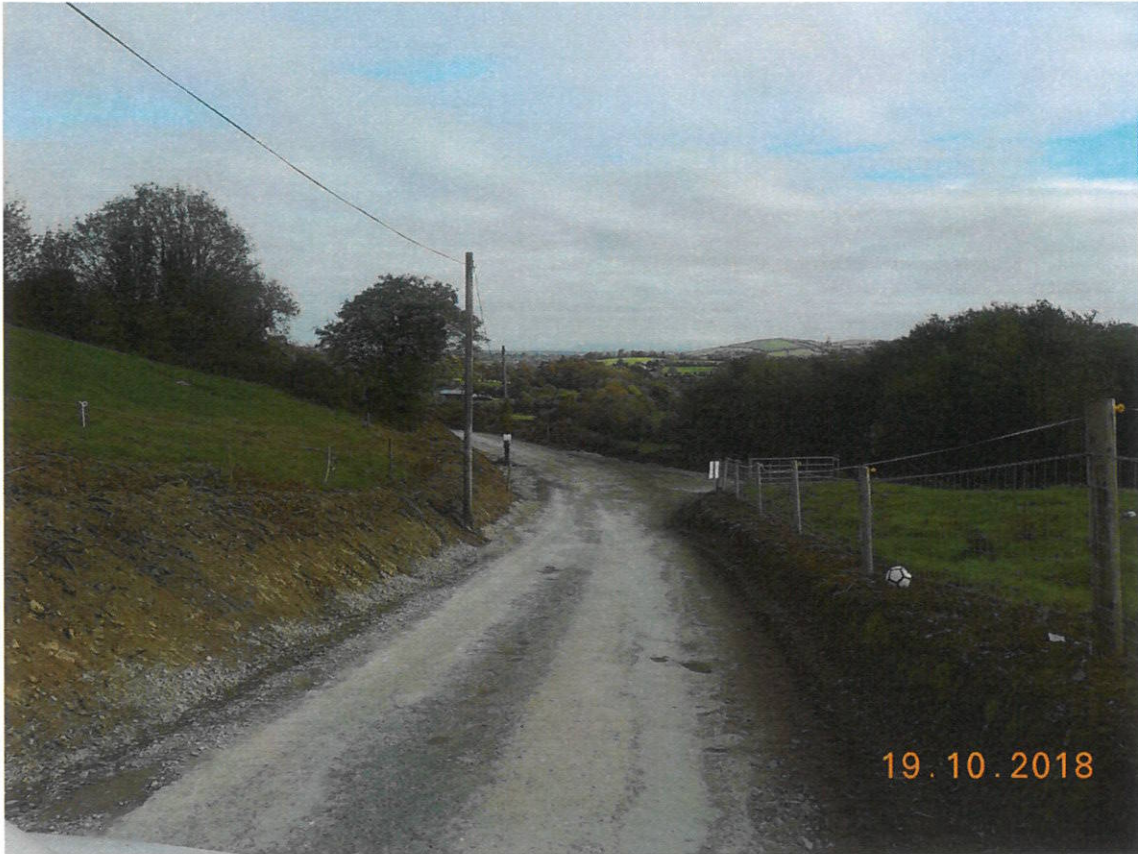
Photograph 2: 19 October 2018, Site Preparations completed on the left hand (north) side of the road at 'Area B' to facilitate safe access and egress of construction traffic to the Mauricetown Wind Farm site, note no duct installation works present on the right hand (south) side of the road.
