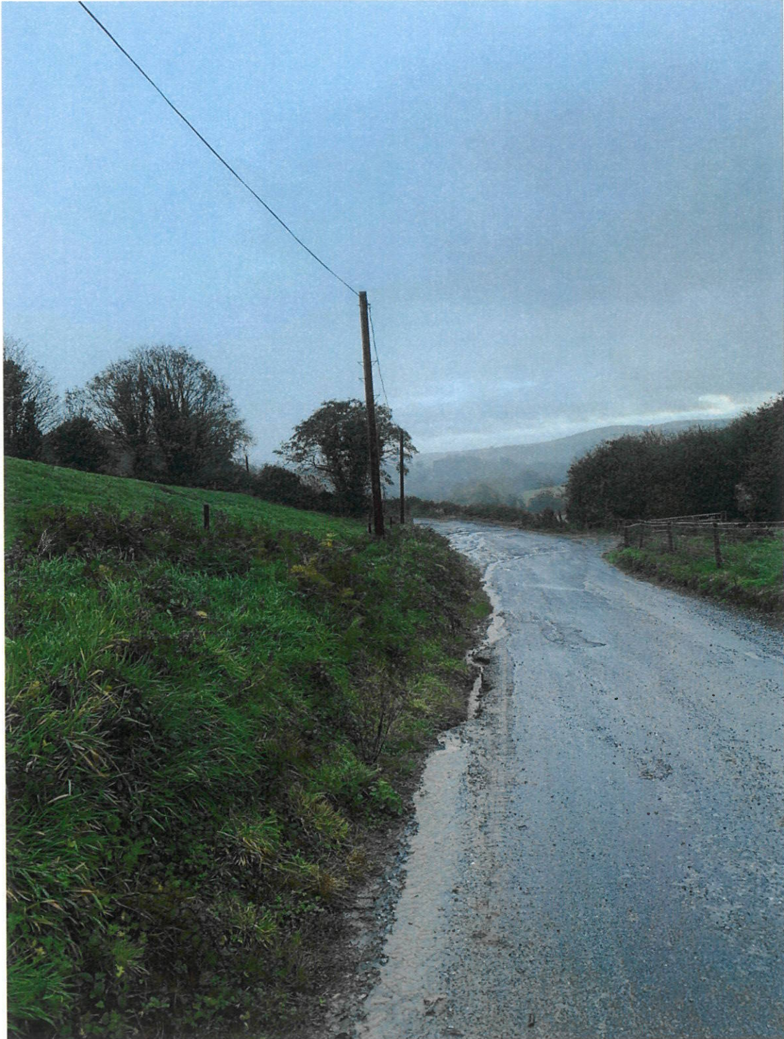
Photograph 4: AFTER - 20 October 2020, Underground duct and cable works reinstated, vegetation on roadside bank recovered to original condition
