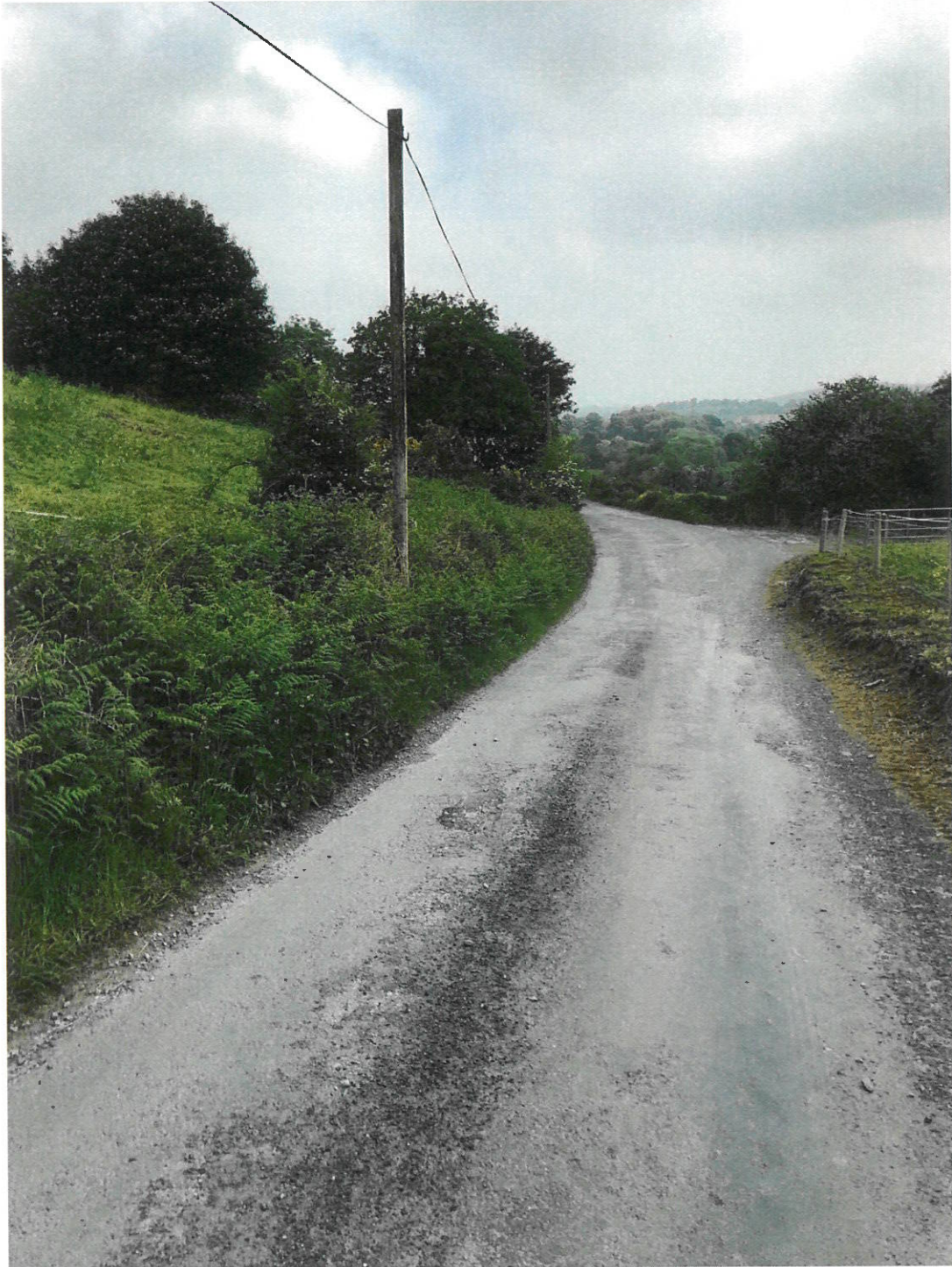
Photograph 1: BEFORE - May 2018, Pre-commencement at 'Area B' looking East. Note that there is NO hedgerow/bank/vegetation on the right hand (south) side of the road and the underground duct has not been installed
