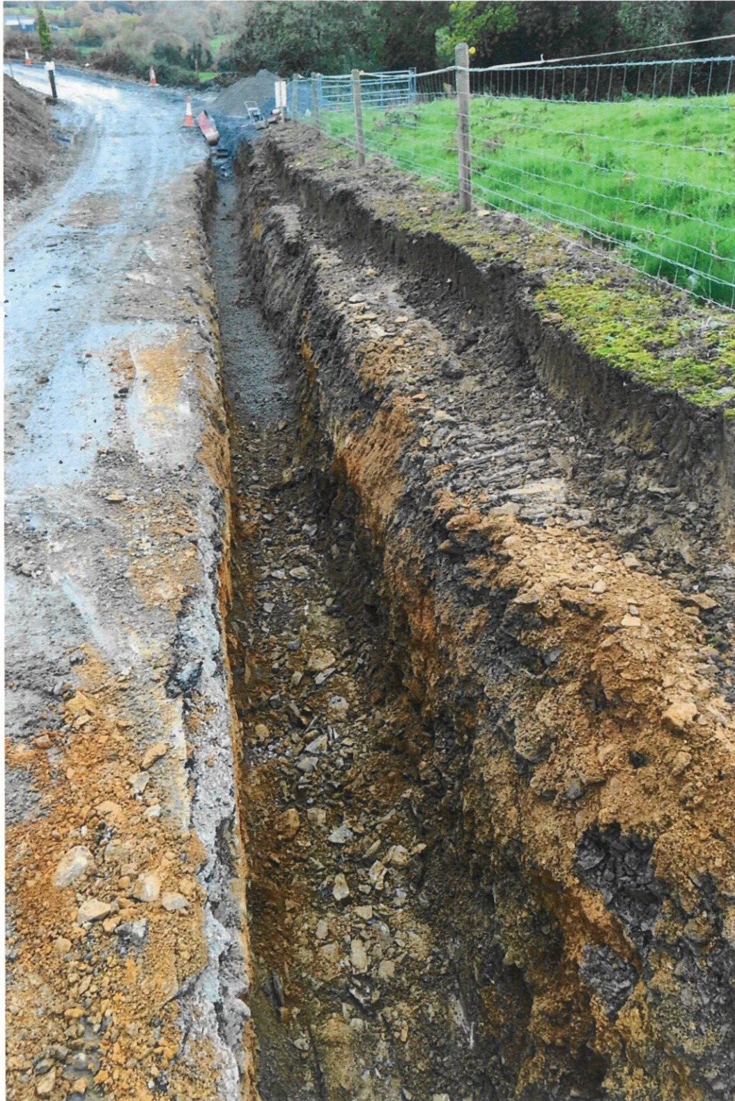
Photograph 3: Week Ending 18 November 2018, installation of underground duct in accordance with Section 5 declaration EC16/59. Note the bituminous bound surface of the road has been cut and imported granular material that pre-existed the trench excavation is visible on the 'outside' face of the trench, i.e. the trench has been cut into the road.
